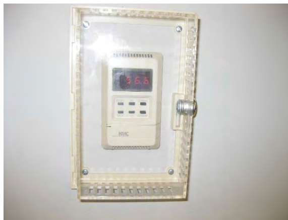
Significant Over-Cooling of
