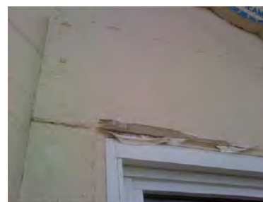
"W1" Recommend sealant around windows
