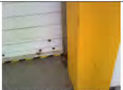
“D17 OH” Recommend weather strip and door sweeps
