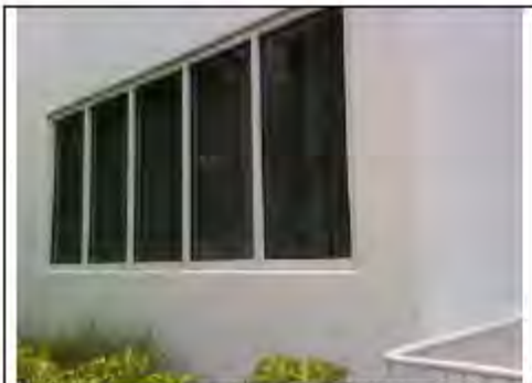
“W1” Recommend sealant
