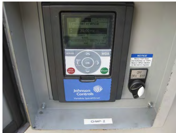
VFD in Bypass Mode (Hand)
