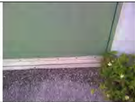
"D9" Recommend weather strip and door sweeps
