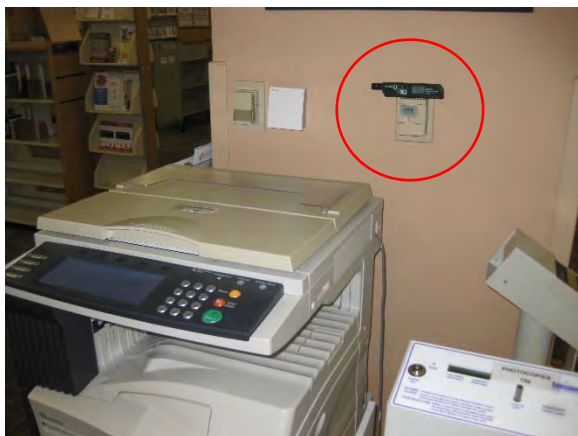
Improper Location of Temperature Sensor Meeting Room
