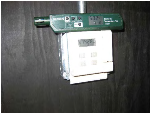
Inaccurate Temperature Sensor
