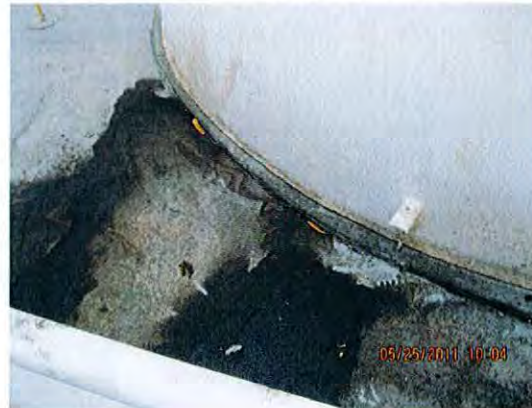
Bottom part of the tank impacted by corrosion
