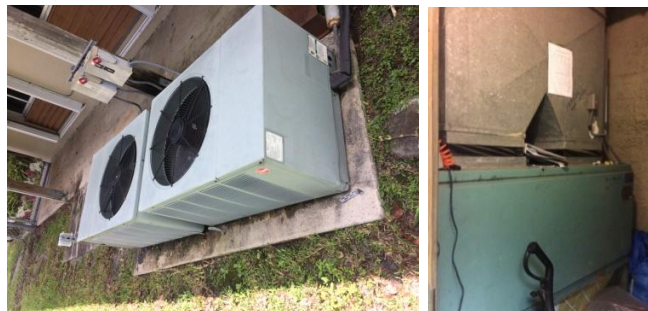
Park Office HVAC
