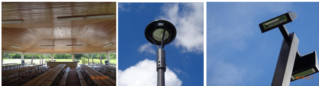
Exterior Lighting Examples
