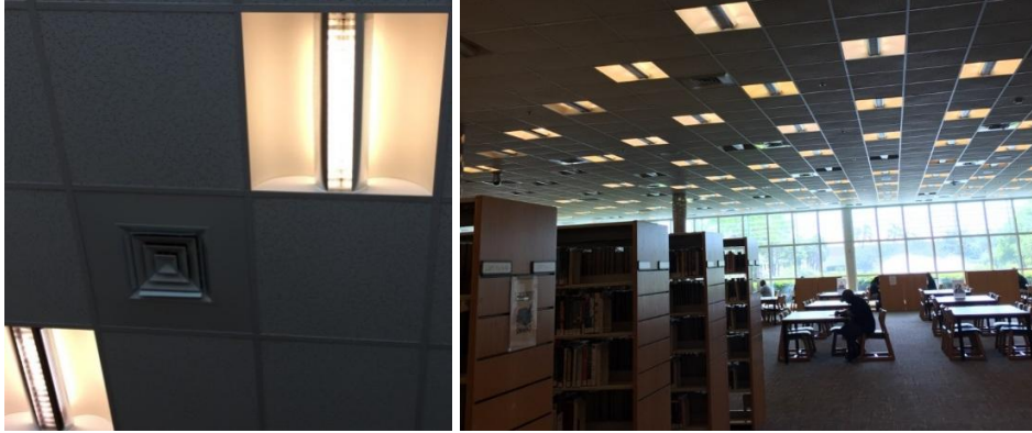
Interior Lighting Examples
