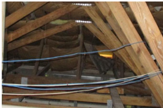
You can see daylight where some fiberglass has fallen away from the roof surface.
