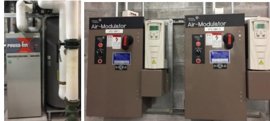
Hot Water System
