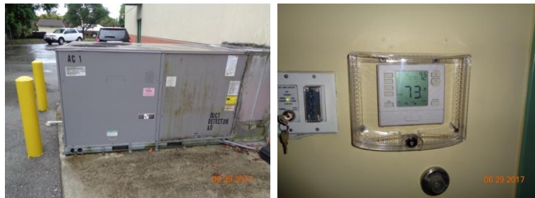
Maintenance Building HVAC
