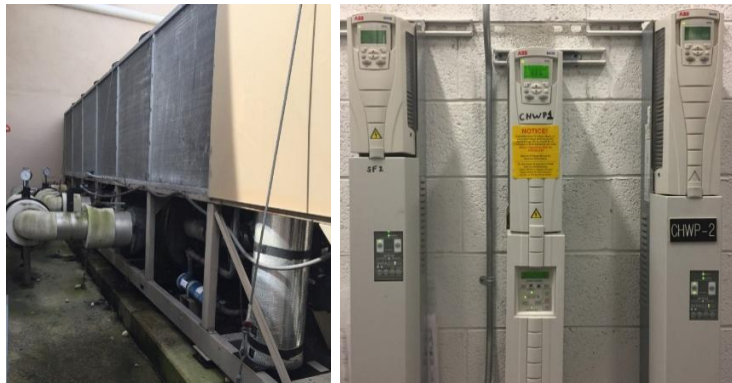
Chilled Water System
