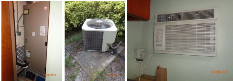
Park Office HVAC
