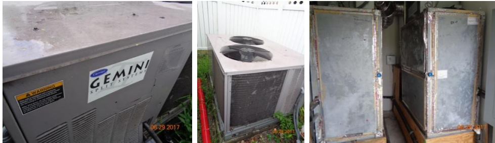
Park Office HVAC
