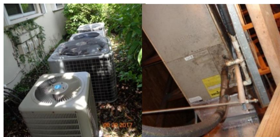
Skeet/Trap Building HVAC
