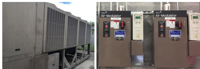
Chilled Water System
