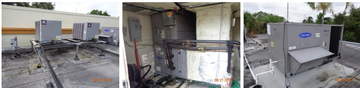
Main Building HVAC
