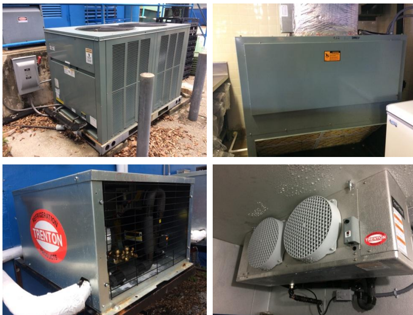
Pool Building Cooling and Refrigeration
