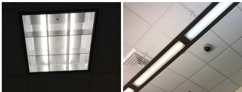
Interior Lighting Examples
