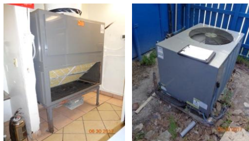
Concessions & Lifeguard Office HVAC
