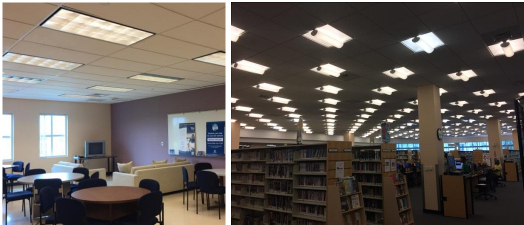
Interior Lighting Examples
