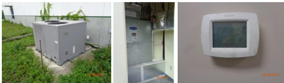
Maintenance Building HVAC
