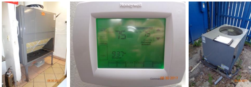
Concessions & Lifeguard Office HVAC
