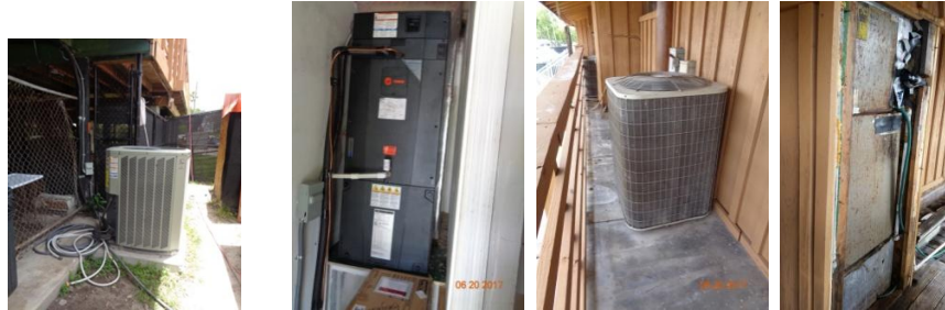
Main Building HVAC
