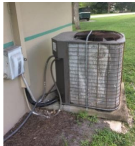
Campground Office HVAC
