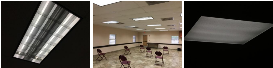
Interior Lighting Examples
