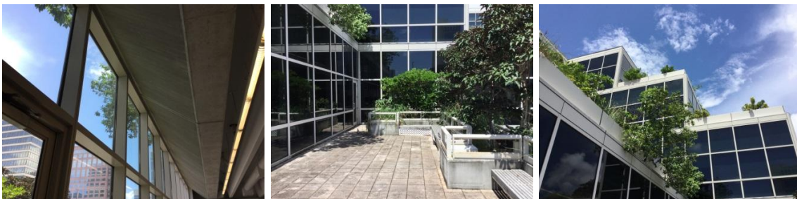
Water Leak Sources
