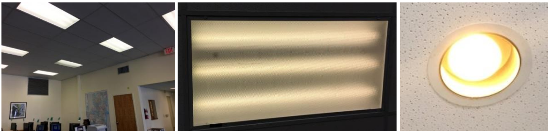
Interior Lighting Examples
