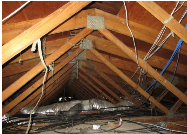
Attic is largely uninsulated.
