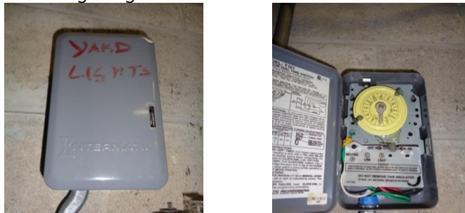
Exterior Lighting Controls
