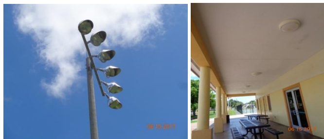
Exterior Lighting Examples
