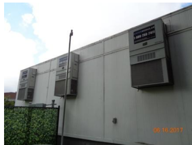
Main Building HVAC
