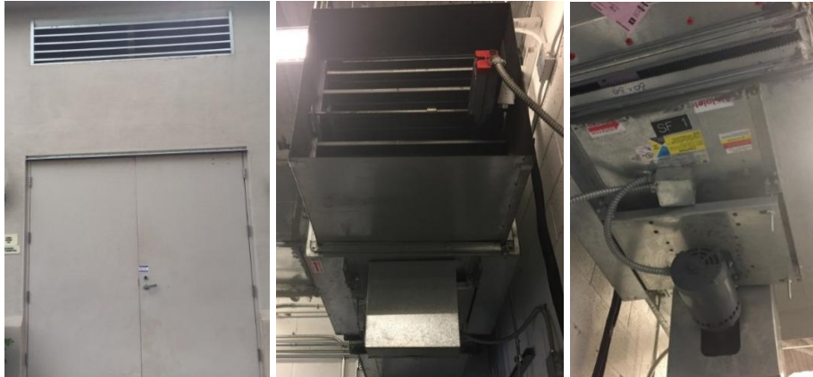
Outside Air for AHU
