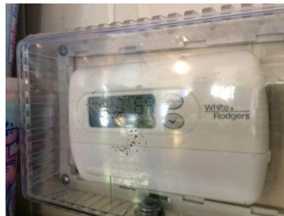
HVAC Controls Equipment
