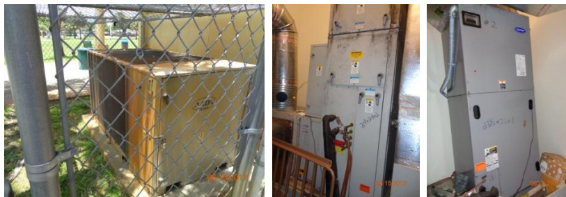
Main Building HVAC
