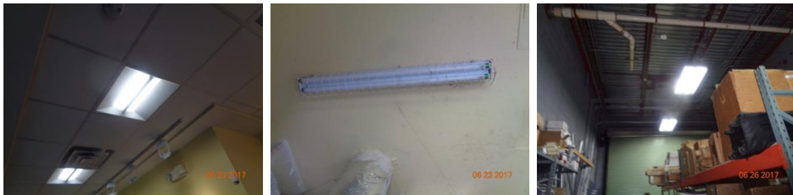
Interior Lighting Examples
