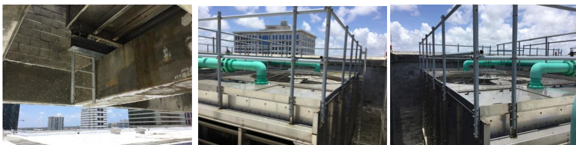
Chiller Plant Cooling Towers
