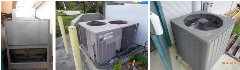
Bike Shop & Sky Rixen HVAC
