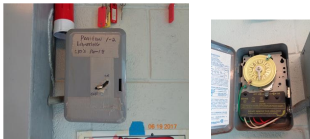
Exterior Lighting Controls
