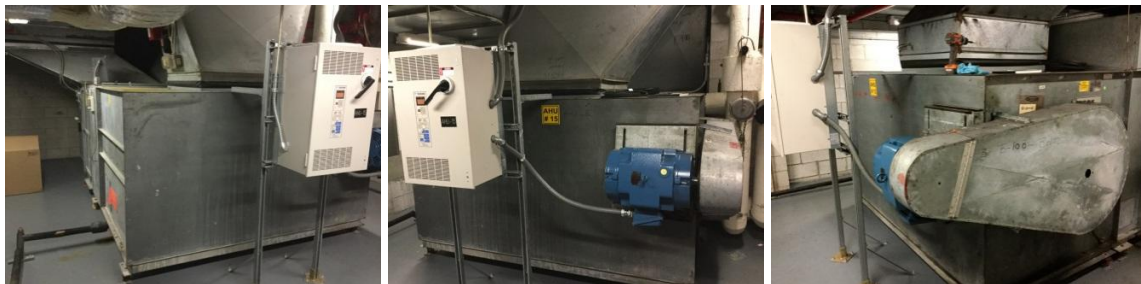
Air Handling Units
