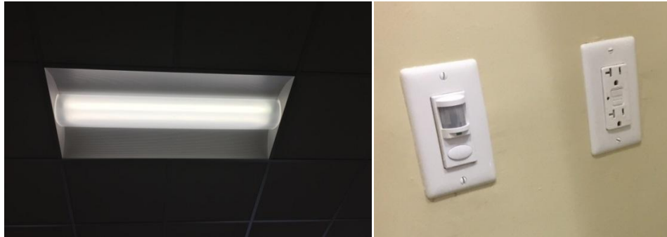
Interior Lighting Examples
