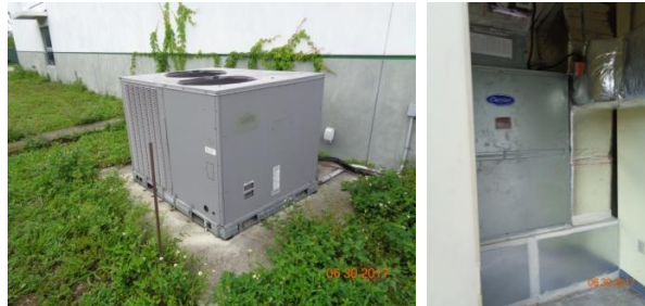
Maintenance Building HVAC
