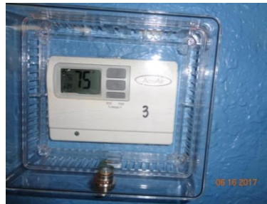
HVAC Controls Equipment
