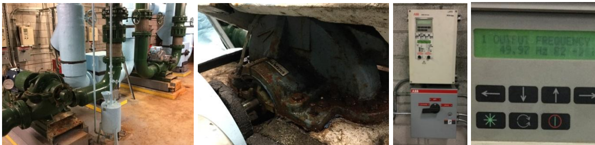
Chiller Plant Pumps
