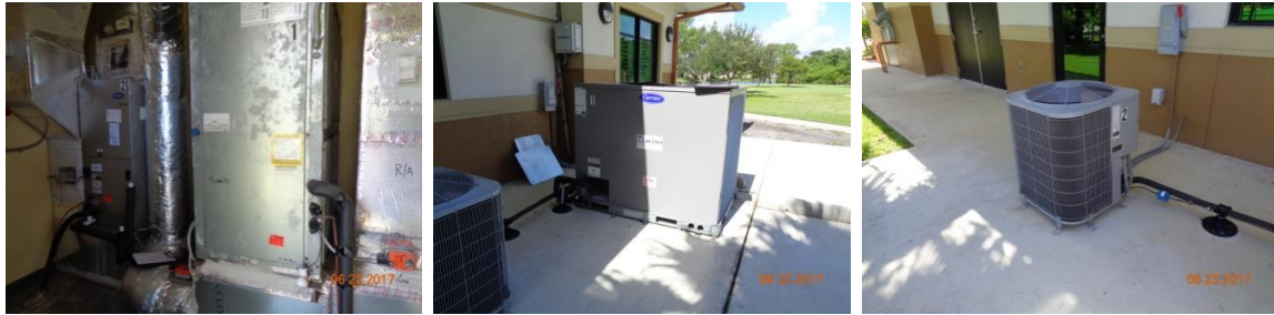
Park Office HVAC
