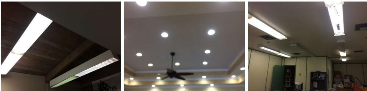
Interior Lighting Examples
