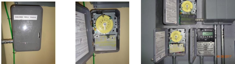
Exterior Lighting Controls
