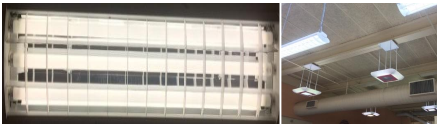
Interior Lighting Examples
