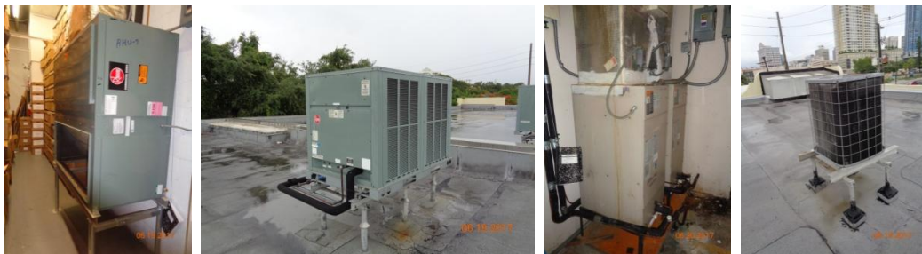
Sate Attorney & Clerk Warehouse HVAC
