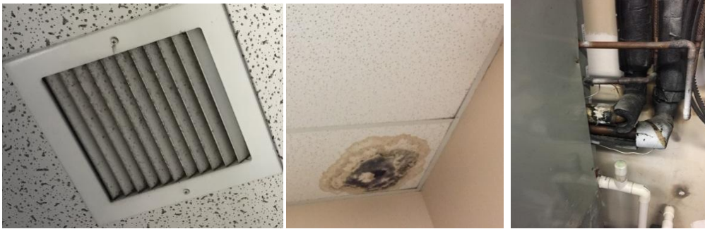
Examples of observed issues
