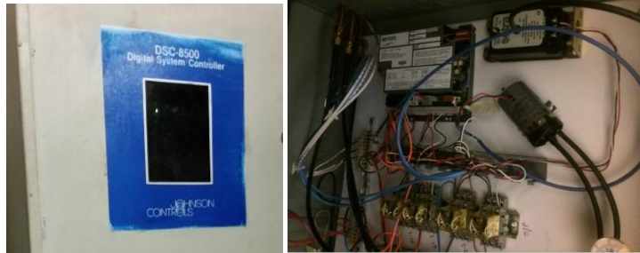
Control System Examples
