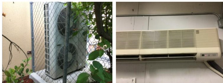
Dedicated Split System
