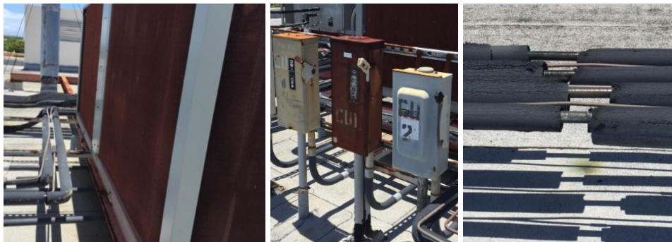
Examples of observed issues
