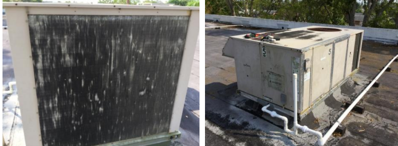
RTU Condition Issues
