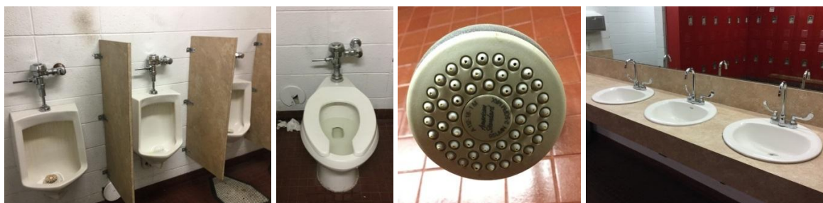
Sample Restroom Fixtures
