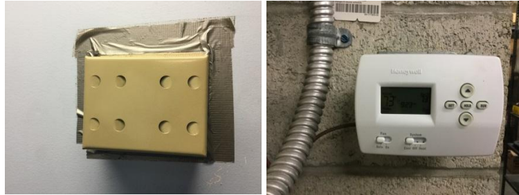
HVAC Controls Equipment
