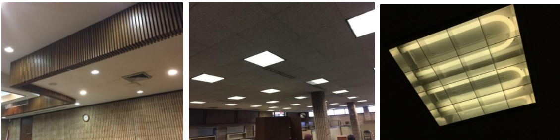
Interior Lighting Examples
