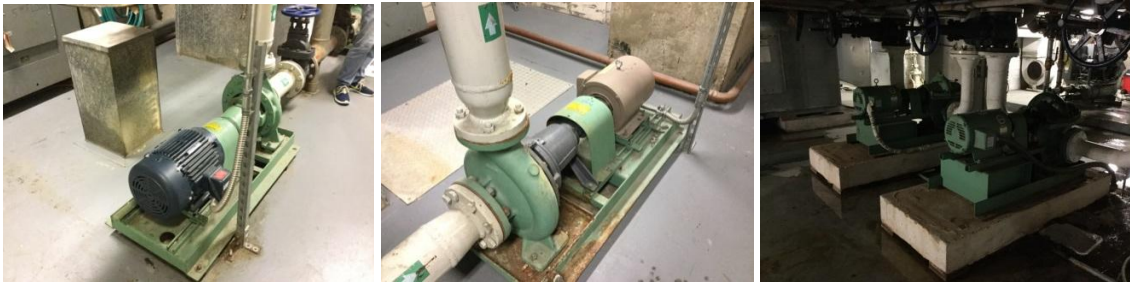
Condenser Pumps Pictured Above
