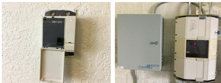
Building Controls Pictured Above
