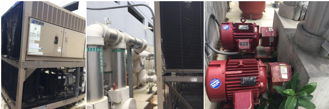
Chilled Water System
