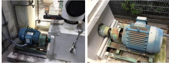
Chiller Plant Pumps
