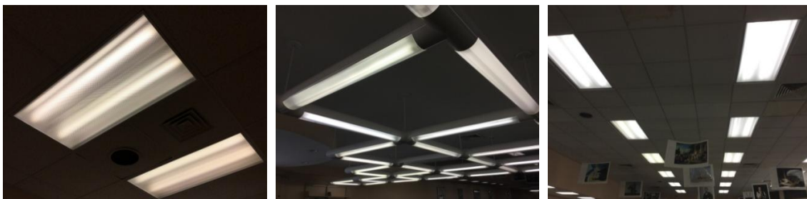
Interior Lighting Examples
