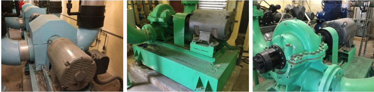
Chilled Water and Condenser Water Pumps
