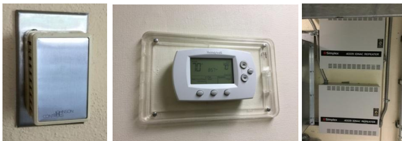
Building Controls Pictured Above
