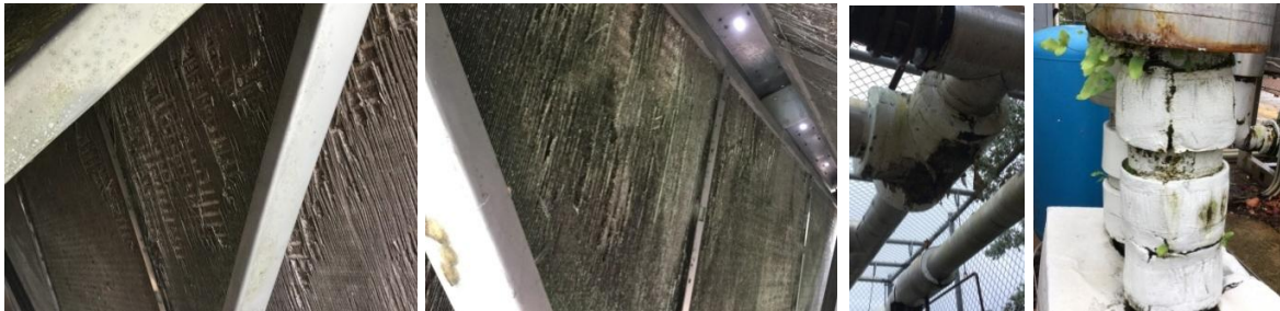
Chiller Plant Observed Issues
