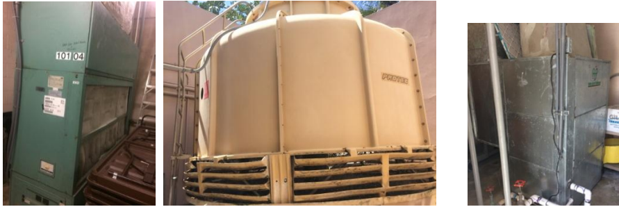
Cooling System Examples
