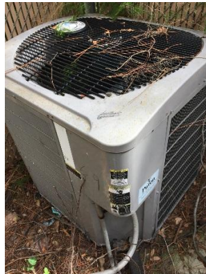
Non-functional Condensing Unit
