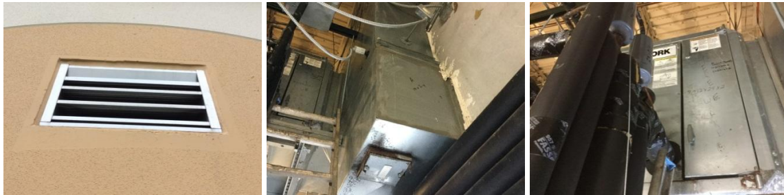
Outside Air System
