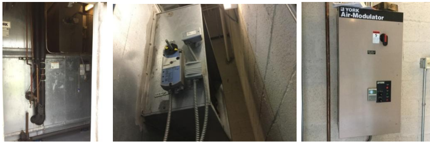
Air Handling Unit Equipment
