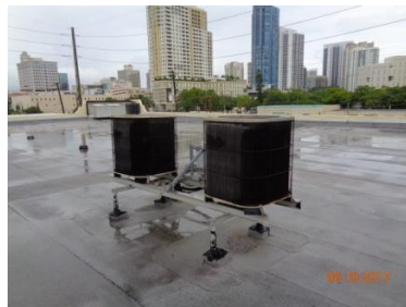
Examples of Observed Issues
