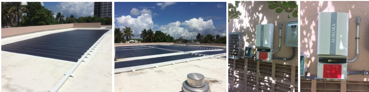
Solar Energy Generation
