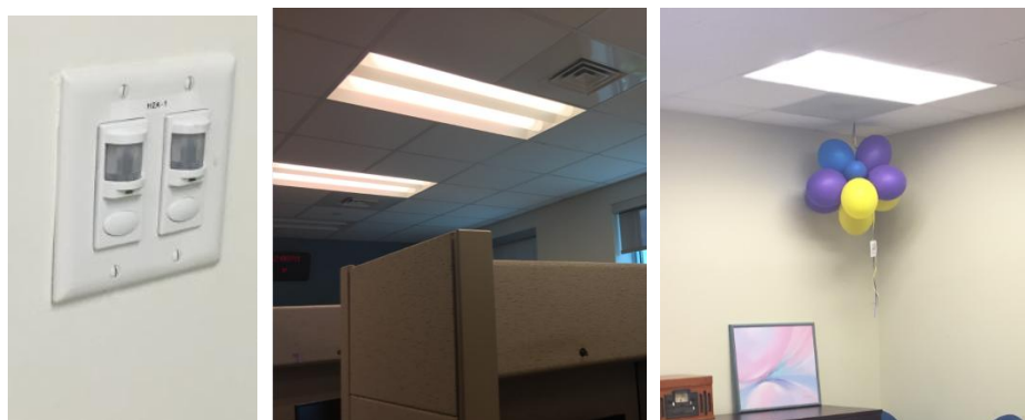
Interior Lighting Examples
