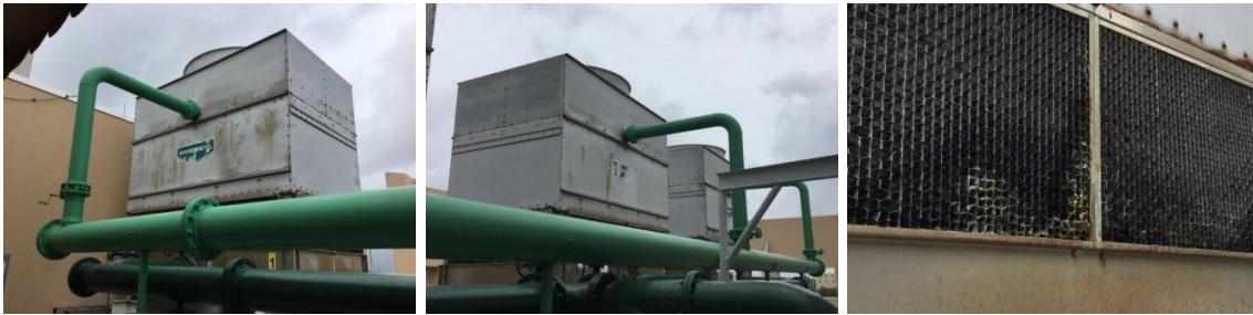
Chiller Plant Cooling Towers
