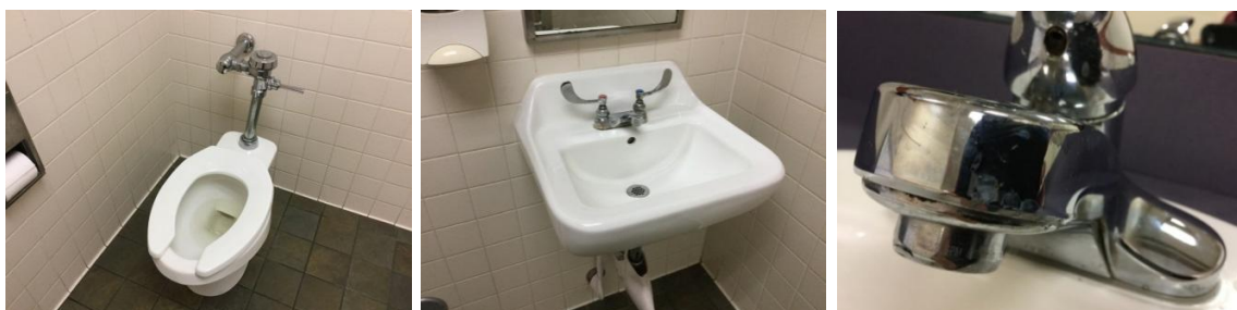
Sample Restroom Fixtures
