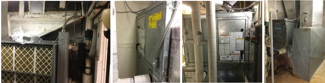
Air Handling Units
