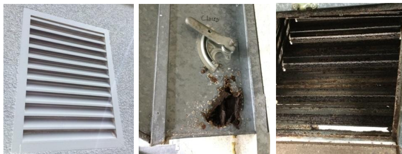
Outside Air for AHU
