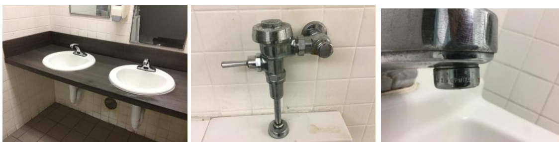
Sample Restroom Fixtures
