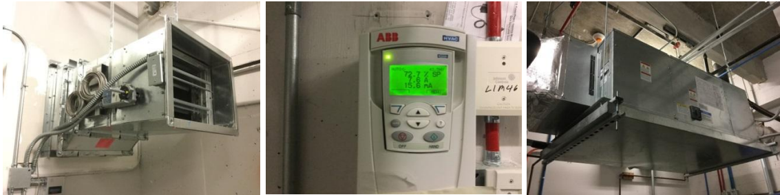
AHU Mechanical Room Equipment
