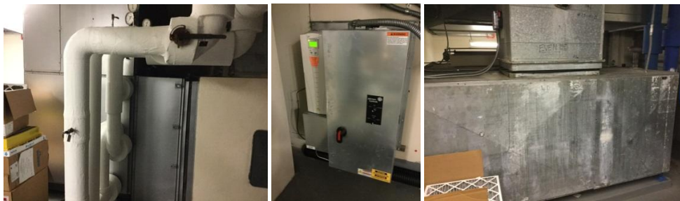
Air Handling Units
