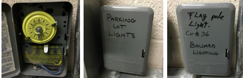
Exterior Lighting Controls
