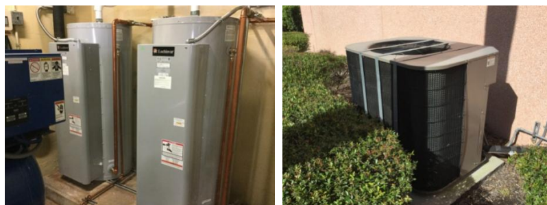
Other Mechanical Equipment
