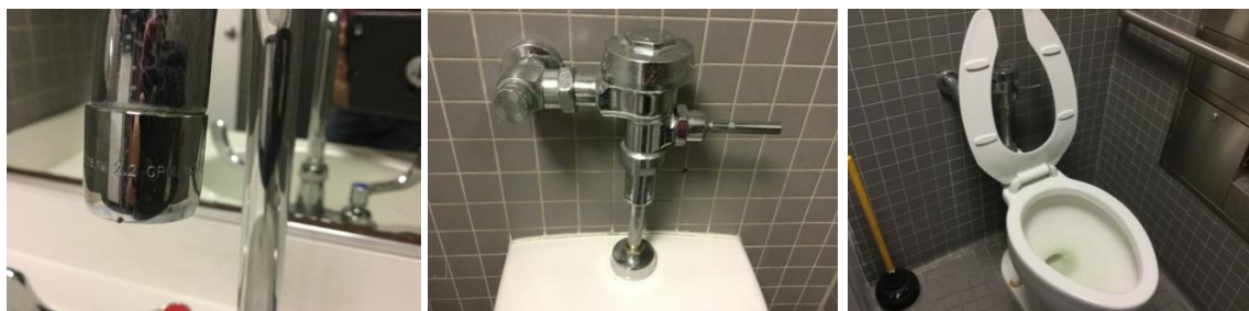
Sample Restroom Fixtures
