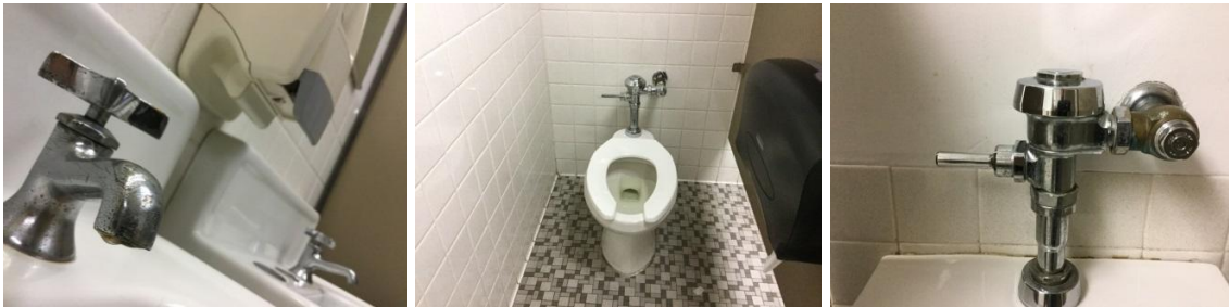
Sample Restroom Fixtures
