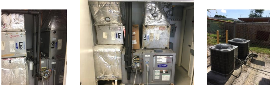
Cooling System Examples
