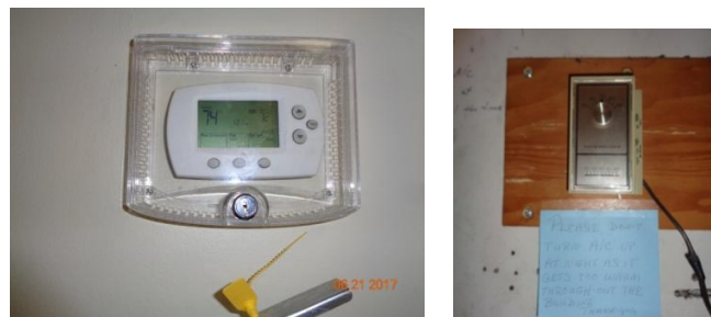
HVAC Controls Equipment
