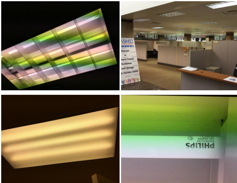
Interior Lighting Examples
