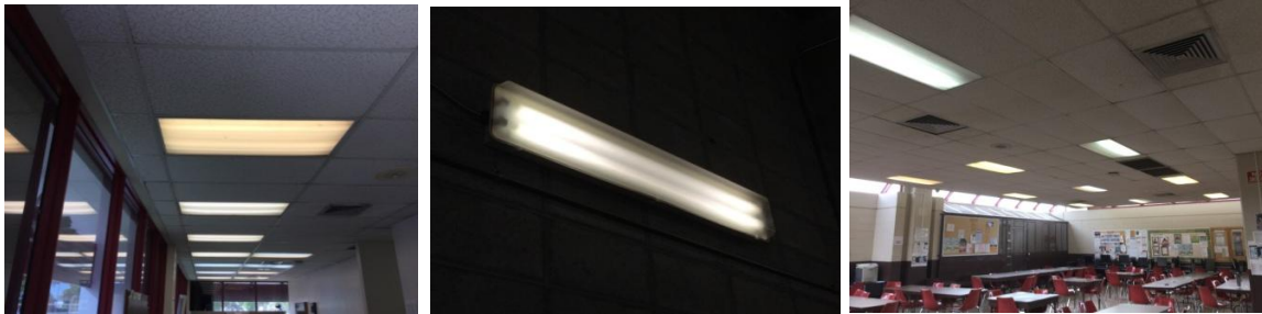
Interior Lighting Examples
