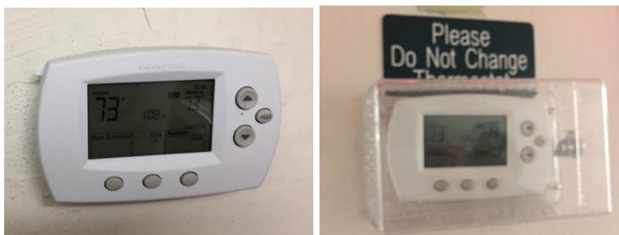
HVAC Control Equipment
