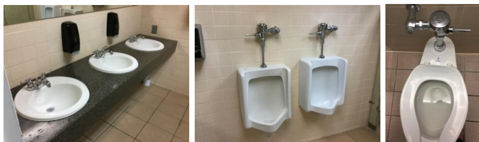
Sample Restroom Fixtures
