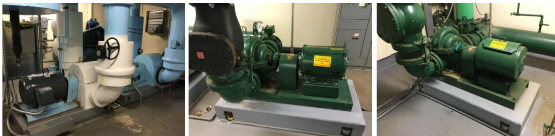
Chiller Plant Pumps
