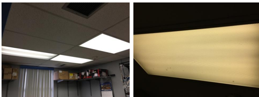
Interior Lighting Examples
