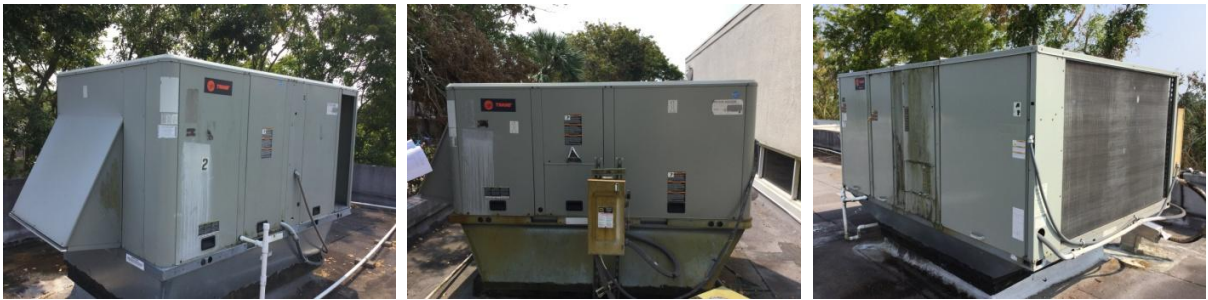
Cooling System Examples
