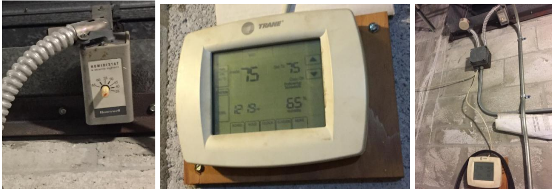
HVAC Controls Equipment
