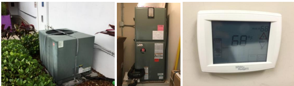
Dedicated Split System
