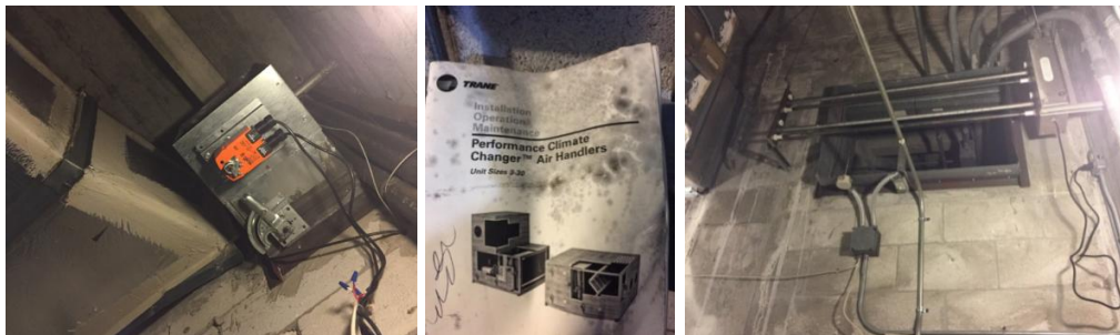
Examples of air handling systems
