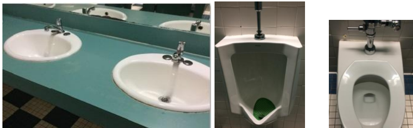
Sample Restroom Fixtures
