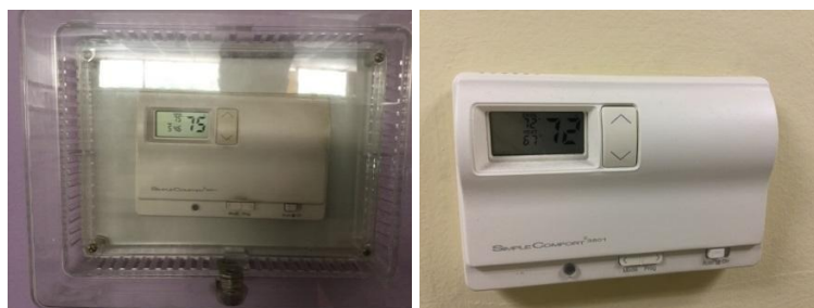
HVAC Controls Equipment
