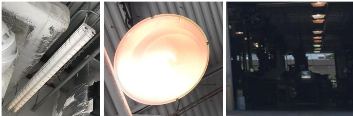
Interior Lighting Examples
