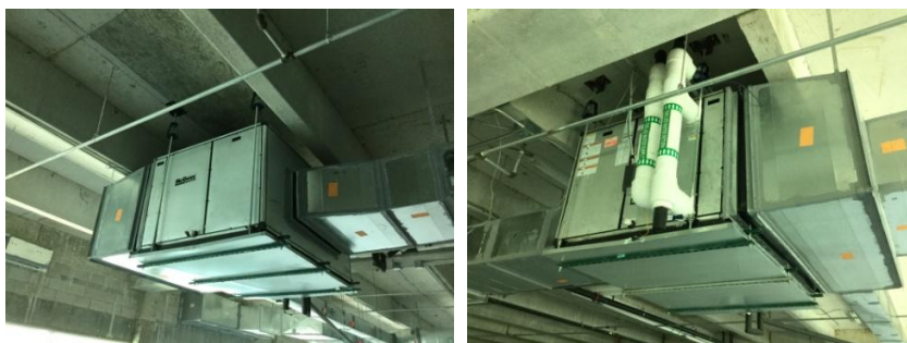
Second Story Air Handlers
