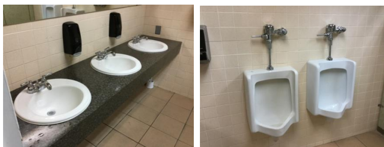
Sample Restroom Fixtures
