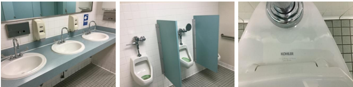
Sample Restroom Fixtures
