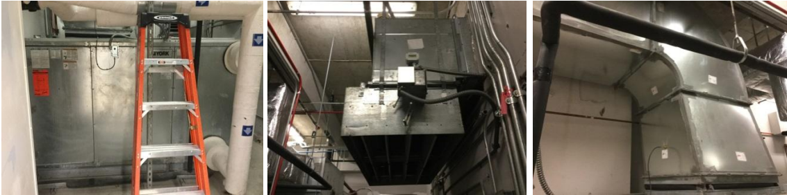
AHU Mechanical Room Equipment
