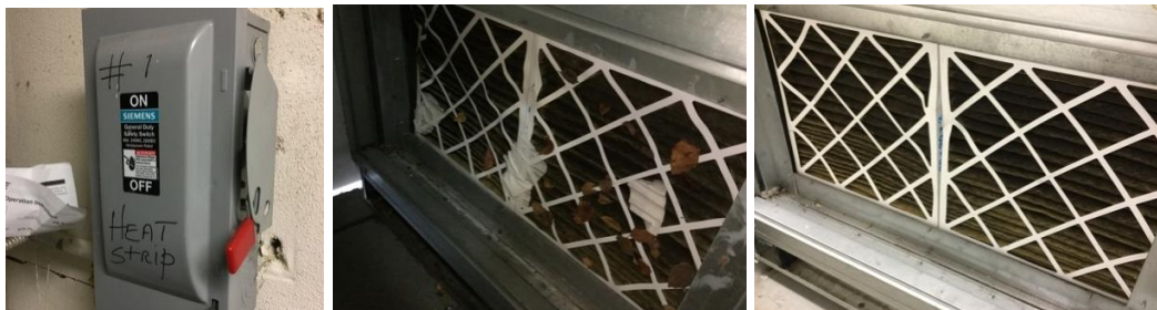
Examples of Observed Issues
