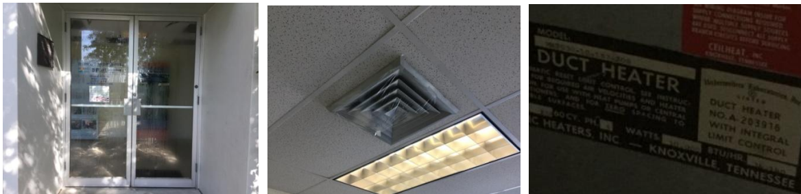
Examples of Observed Issues
