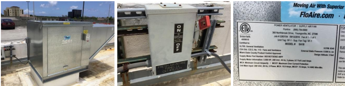
Supply Air Intake
