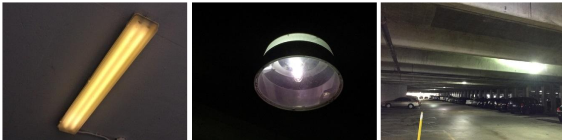
Interior Lighting Examples – East Garage
