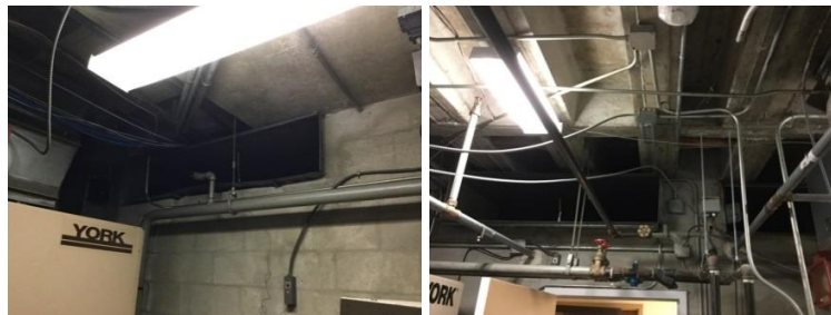
Mechanical Rooms Pictured Above
