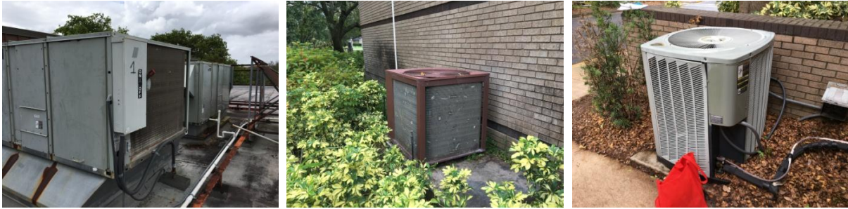
HVAC Controls Equipment
