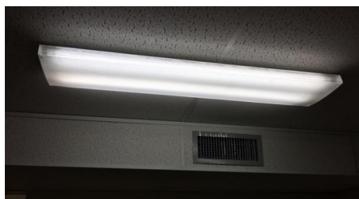
Interior Lighting Examples
