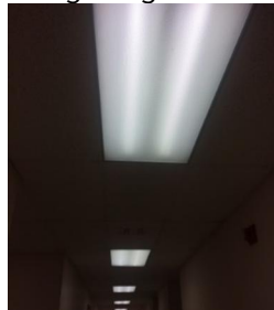
Interior Lighting Example
