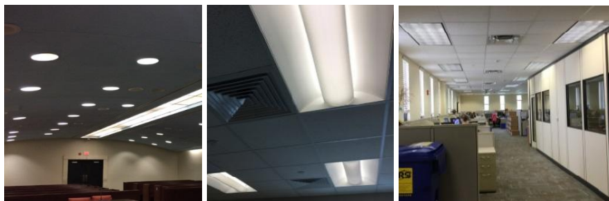
Interior Lighting Examples
