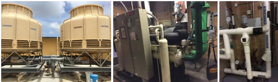
Chilled Water System
