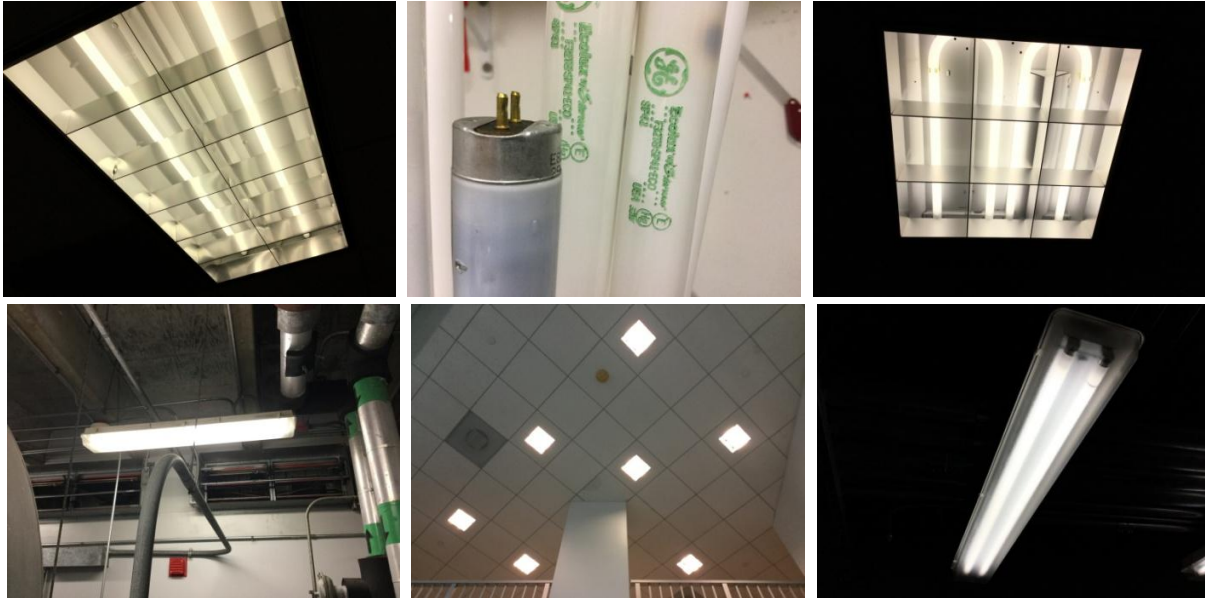
T8 Interior Lighting
