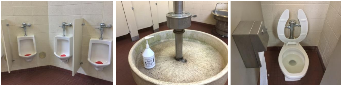
Sample Restroom Fixtures
