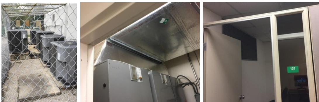
Air Conditioning System
