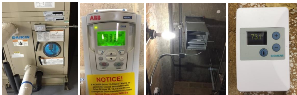
HVAC System Examples
