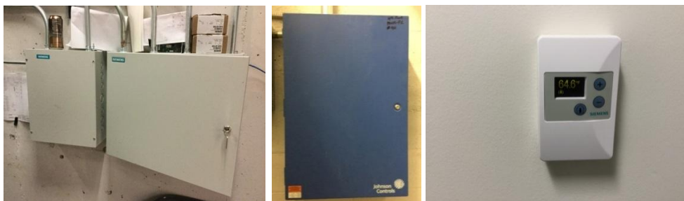
HVAC Controls Equipment
