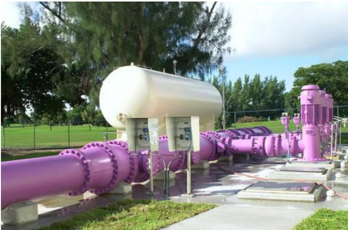
Pompano Beach wastewater reuse facility
