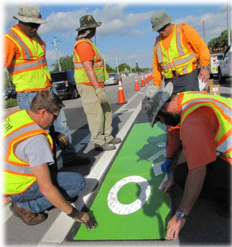
Installation of a green bicycle lane on Bailey Road, another Broward Complete Streets project.
