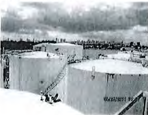
Top area impacted by corrosion
