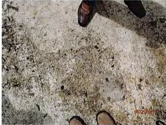
cracked/peeling sealant in containment structure
