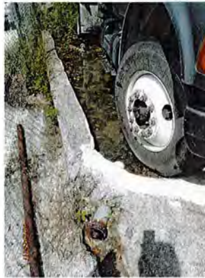
drainage valve in truck park area
