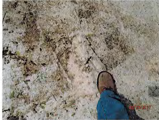
cracked/peeling sealant in containment structure
