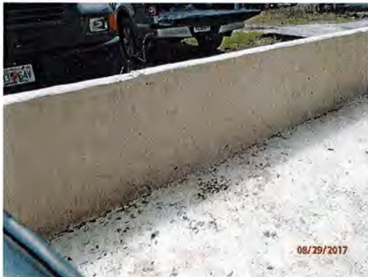
cracked/peeling sealant in containment structure
