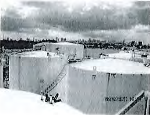
Top area impacted by corrosion
