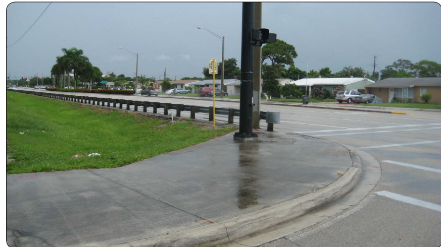
Figure 4.4.1b - Photo - Guardrail at Bus Stop - Undesirable Layout. Sheridan St. and NW 70th Terrace
