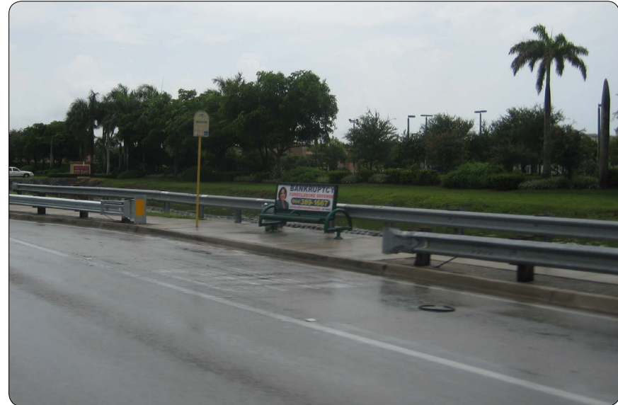
Figure 4.4.1a - Photo - Guardrail at Bus Stop - Recommended Layout. University Blvd and Taft St.
